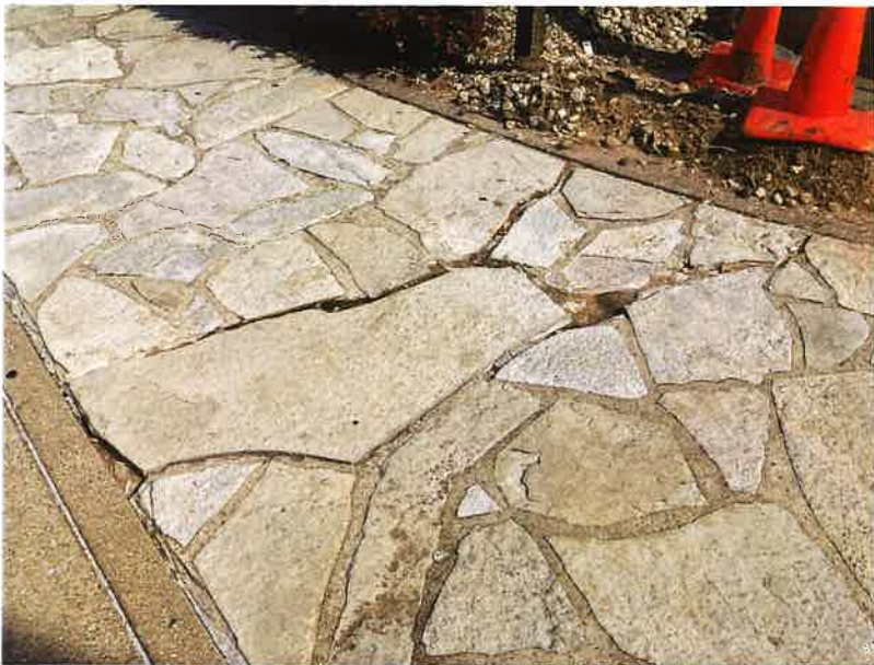
Missing mortar / loose stones
