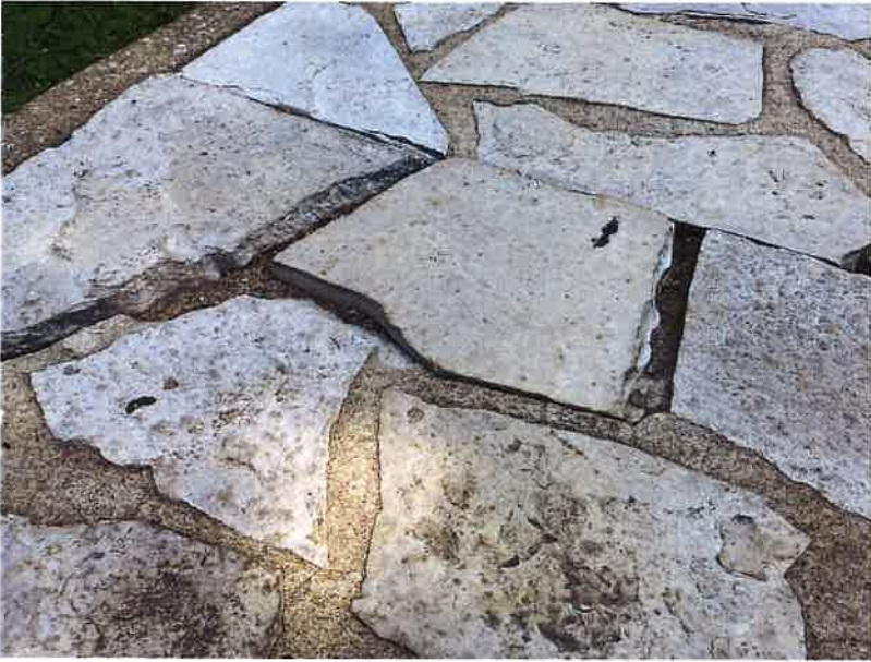
Missing mortar / loose stones
