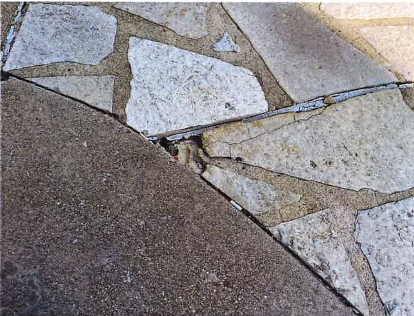
Missing stone and mortar
