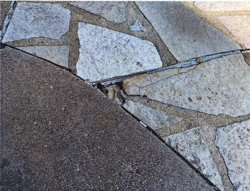
Missing stone and mortar
