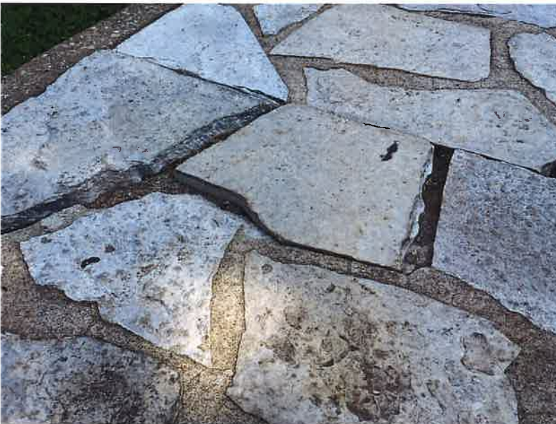
Missing mortar / loose stones
