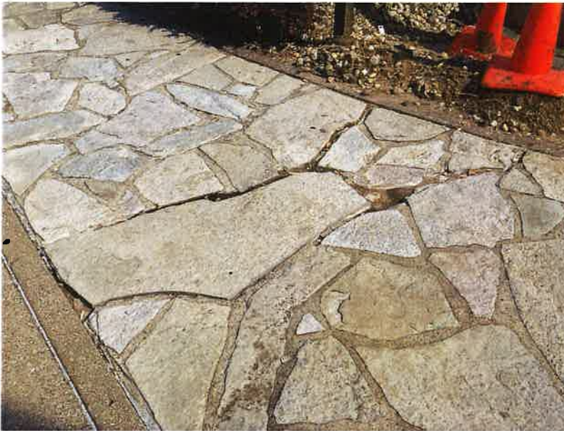
Missing mortar / loose stones
